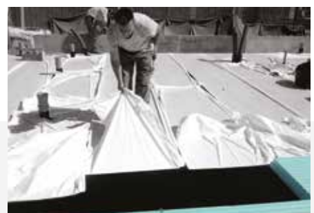
Step by step, the protective foil is removed from the two-sided self-adhesive waterproofing membrane FIBRANhydro SEISMIC T-1,8 sk/sk.
