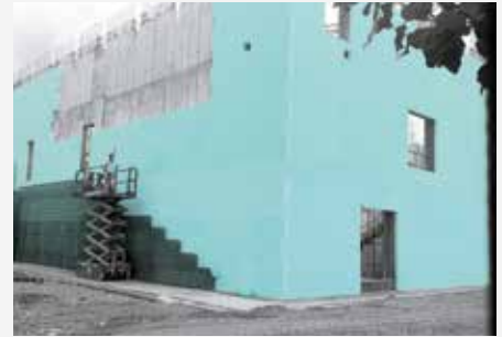
FIBRANxps MAESTRO as sandwich insulation; visible white concrete outer wall construction phase.
