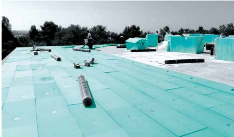
Increasing the roof slope with FIBRANxps INCLINE and simultaneous flat roof thermal rehabilitation.
