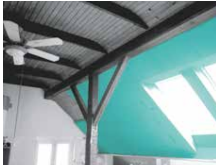
Interior thermal insulation using FIBRANxps ETICS, surface protected with coatings of thin-layered render and paintwork.
