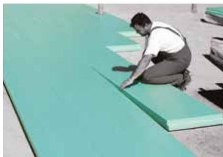
Before pouring the levelling concrete and laying the first layer of FIBRANxps (400-L, 500-L, 700-L) thermal insulation, special attention is given to installation pipes.
