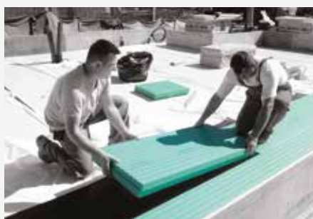
FIBRANxps SEISMIC boards are laid carefully and precisely on the adhesive waterproofing surface.
