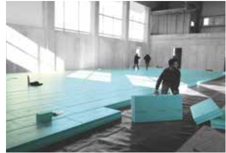
Fitting of thermal insulation FIBRANxps 500-L underneath foundation slab of multi-functional building.
