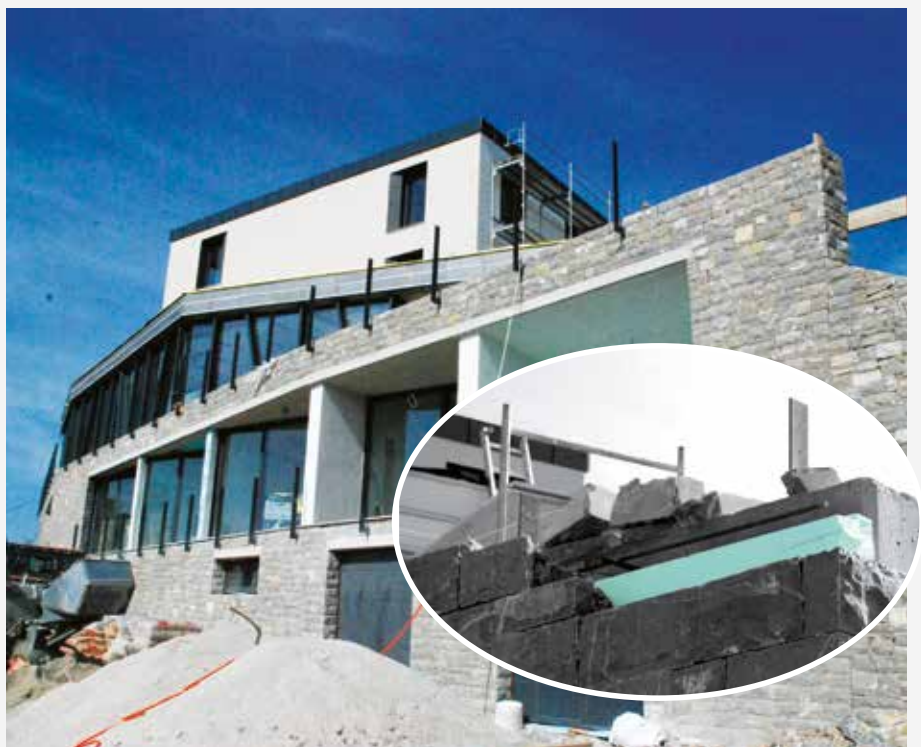
Stone cladding of a hotel building facade with load-bearing insulation FIBRANxps ETICS BT-I, to which natural stone is glued with a special procedure.
