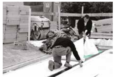
Two-sided self-adhesive waterproofing FIBRANhydro SEISMIC T-1,8 sk/sk is laid onto the first layer of the suitably thick and loadbearing FIBRANxps thermal insulation panels.
